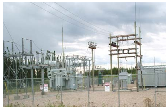
Typical 144-25 kV Substation
